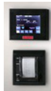
Trinity Control Panel /Printer Arrangement
